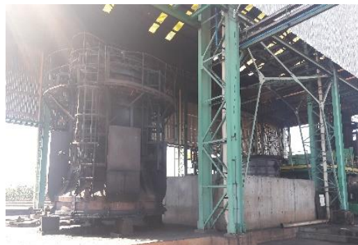
Project Supported Metallic kiln ("forno-container")
