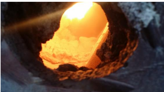
Burner running on natural gas
